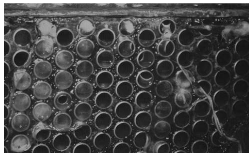
Figure 8. Microbiological growth on heat exchanger tubes.
